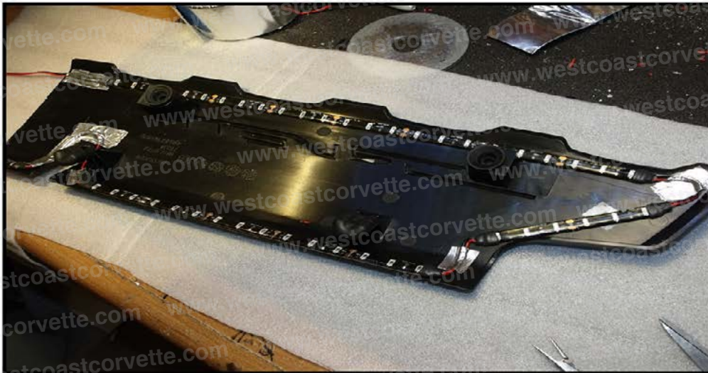
This shows the drivers side location of the led strips. First, wipe down the mounting area with degreaser then alcohol swabs. Next, cut the very top off the adhesion promotor pack. Squeeze the excess fluid back into the packet as you remove the sponge. Apply a thin coat to the area where the strips mount. Let dry for a 2 minutes. Apply the strips within 1 hr.
